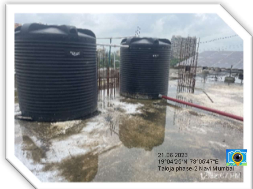
Overhead water tanks
