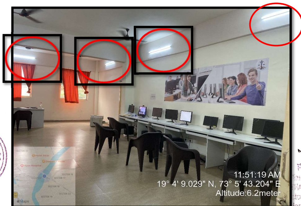
Figure 2: Example of lack of proper lighting management
